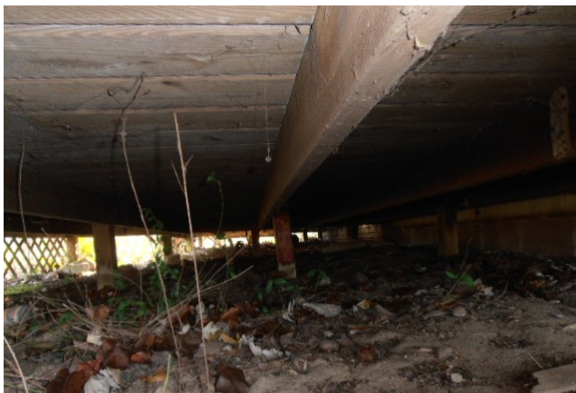
Overspanned Deck Joists
